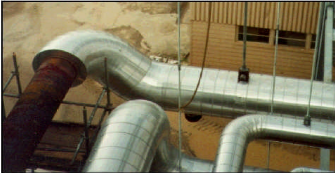
Hot Supports in a Plant Environment
