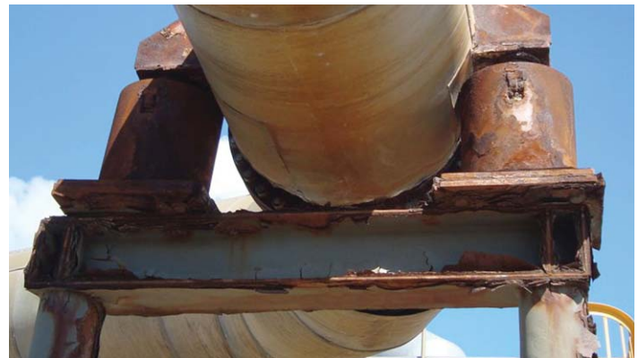
NON PT&P Painted Support 8 Years In-Service in Louisiana
