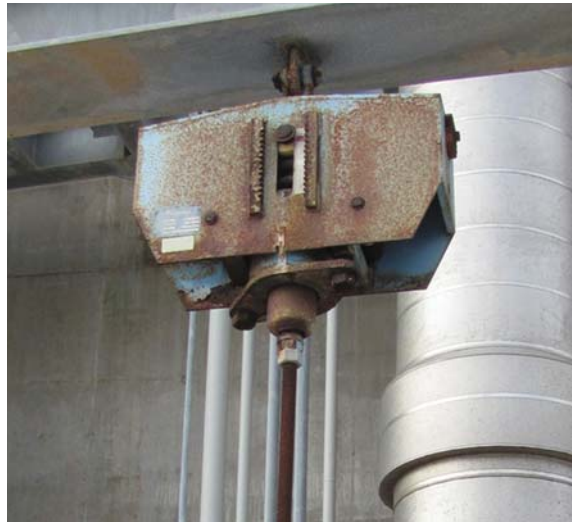
NON PT&P Painted Support 8 Years In-Service in Texas Salt Air From Gulf Coast
